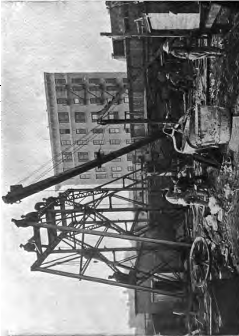
PLATE 212.—Contract 65, City Aqueduct. Erection of steel headframe over shaft, which was sunk part way with derrick after which permanent plant with hoist and headframe was erected for remainder of shaft sinking, etc.
